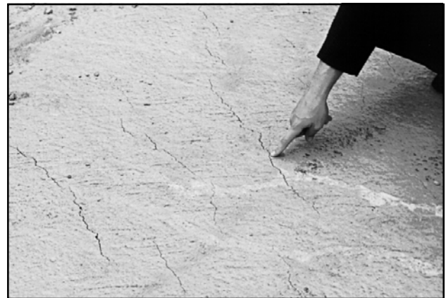
Plastic Shrinkage Cracks
