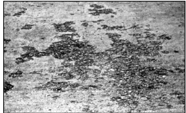
Scaling concrete surface
